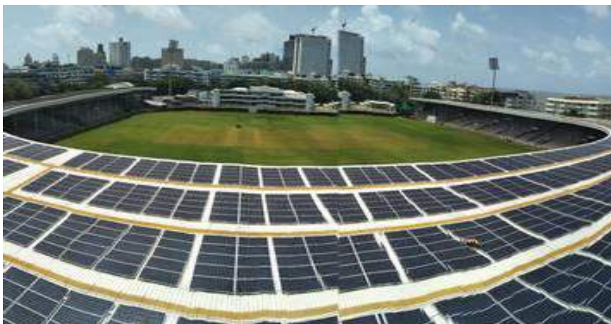
Figure 6.1: Solar rooftop of Brabourne Stadium, Mumbai
